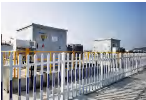
厂址外右侧光伏箱变
